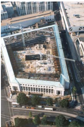
An aerial view of restoration work on the Postal Square Building in the early 1990s. There is no roof on the building; the large hole in the center marks the museum's atrium, where the large skylight is now.
